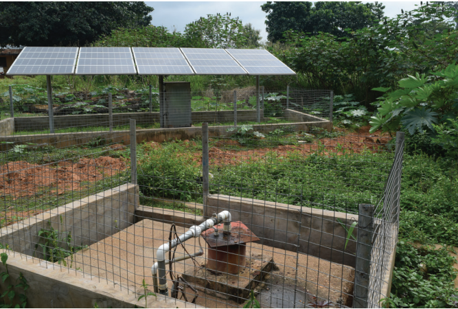
A photovoltaic installation in Ananekrom, Ghana.
